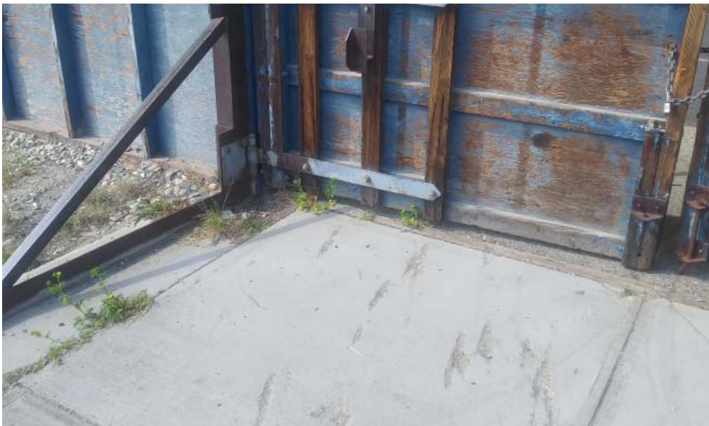
Zamboni gate needs replacement.
